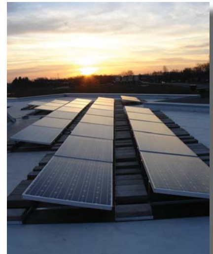
Twenty-seven solar panels and two solar thermal panels line the roof of IMPA's building. The Agency invested in renewable energy projects to provide a demonstration for member communities. The project complements agreements in member communities that allow consumers to enter into net metering contracts.
