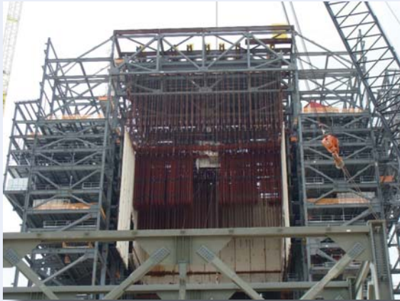
Prairie State Unit 1 Boiler Tube
