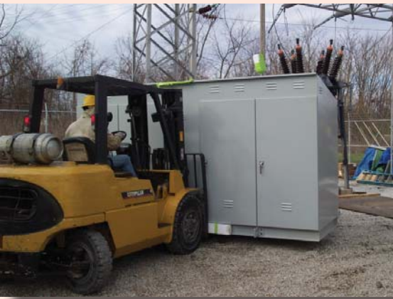
A contractor places a new control cabinet at a substation in Lebanon.
