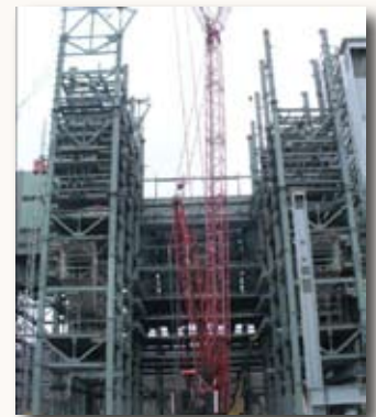
Structural steel is being erected for the boiler at Trimble County Unit 2.
