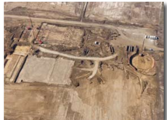
An aerial view of the Prairie State Energy Campus shows the progress that has been made thus far on the project.
