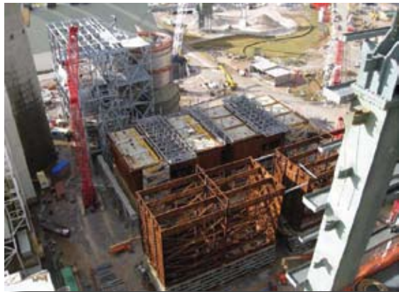
Aerial view of Trimble County Unit 2 Air Quality Control Systems
