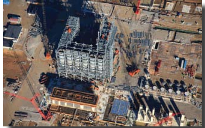
Aerial view of Prairie State Unit 1 boiler structure
