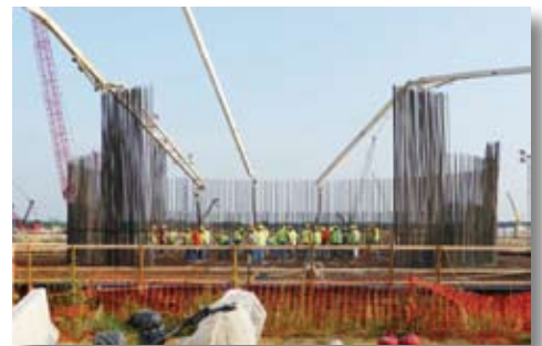
Crews place concrete for the chimney foundation at the Prairie State Energy Campus.
