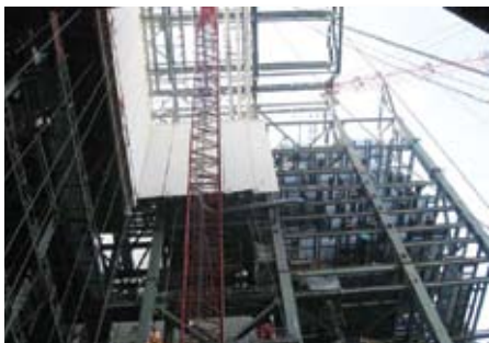
Bechtel rigs the upper furnace sidewalls of the boiler at Trimble County Unit 2.
