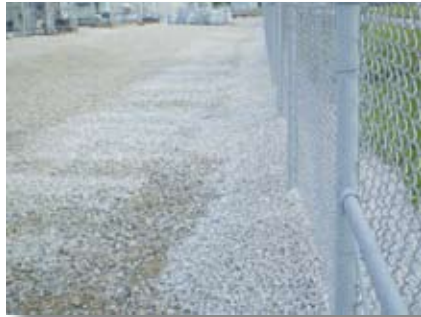
Working with ISC, Tell City Electric constructed berm installations at three of its substations to contain any spills should they occur.
