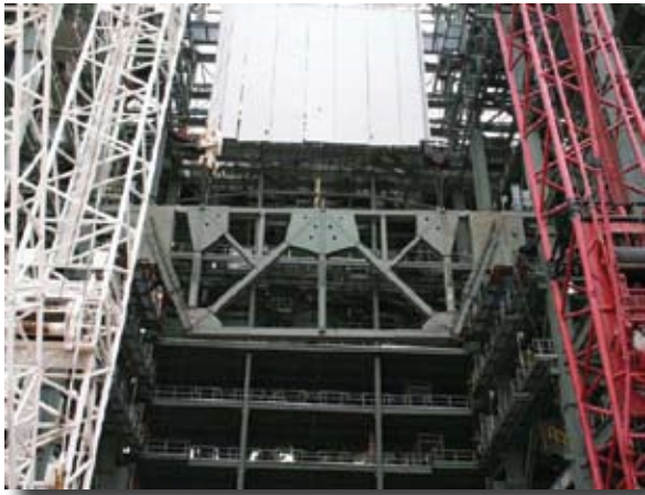
Bechtel has installed the first of two heavy trusses at Trimble County Unit 2.
