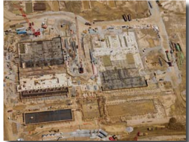
This May 2008 aerial photo of Prairie State shows the ongoing foundation work currently being performed at the site for Units 1 and 2.
