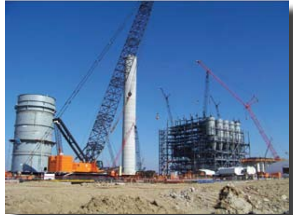
Prairie State Unit 1 with sixth coal silo at left
