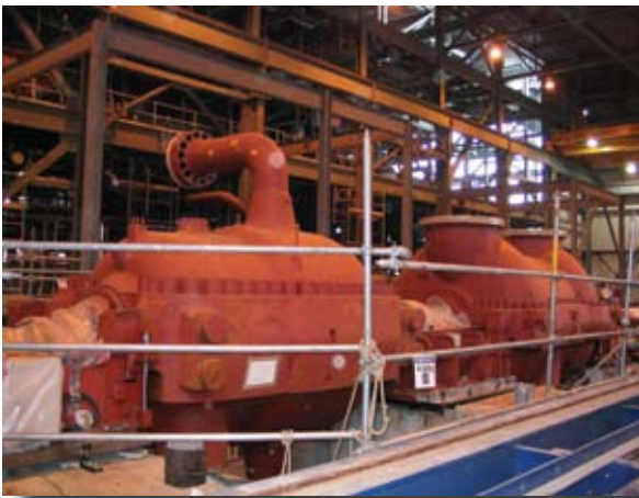
Trimble County Unit 2 high and intermediate pressure turbines
