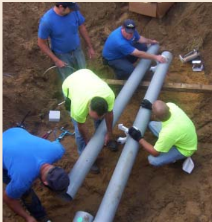
Bremen utility crews work to install conduits underneath a railroad to carry service from one side of Bremen to the other.
