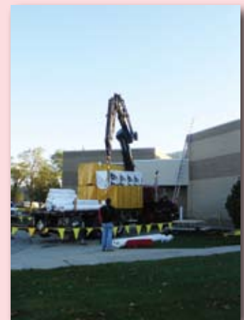
C.E. Reeve, a local contractor, delivers materials for a new, energy efficient roof at IMPA's headquarters.
