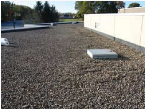
IMPA's rock ballast, rubber roof is being upgraded to a new material that is resistant to punctures, tears and abrasive elements and is more energy efficient.
