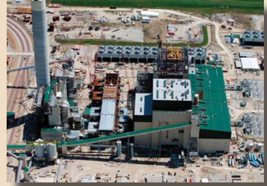
A bird's eye view of the Prairie State Energy Campus looking East with Unit 1 in the foreground.
