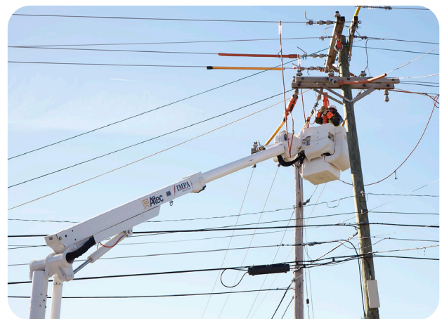
Lineworkers are on the frontlines of the COVID-19 pandemic to provide a reliable supply of electricity.
