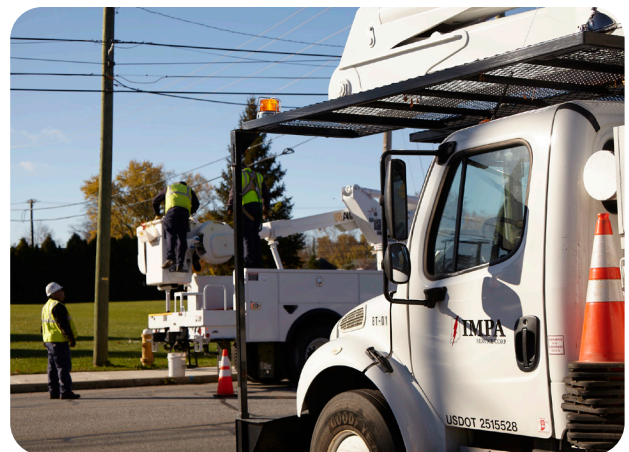
IMPA’s crew of lineworkers continue working in the field to ensure essential access to power.
