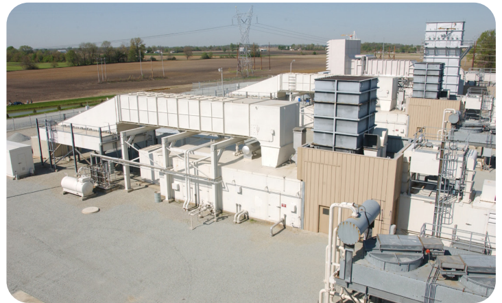
IMPA wholly-owns seven combustion turbines that generate electricity using natural gas, such as this one in Anderson.
