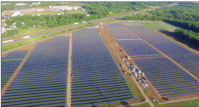
The photo above shows the progress of the 7.44 MW Richmond 2 Solar Park as of June 2018.
