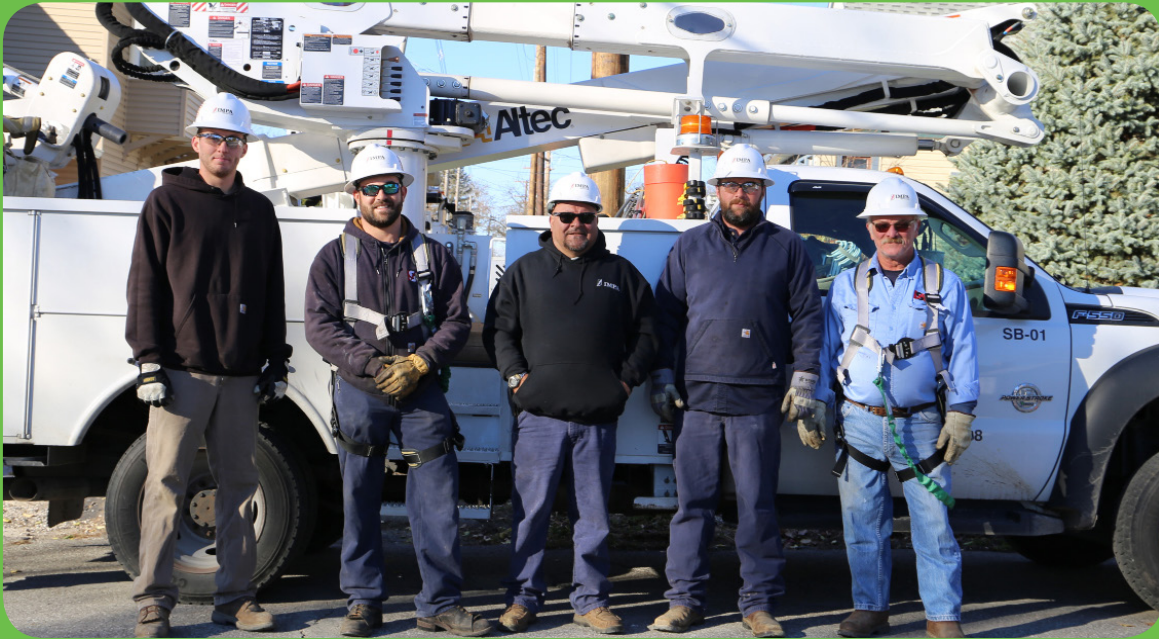
IMPA Service Corp linemen work on newly placed power lines for a community in the Dedicated Services Program. Spiceland is one of several IMPA member communities that benefits from the Dedicated Services Program, which aims to maintain safe and reliable electric service.
