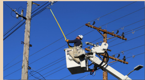
IMPA Service Corp employees work on newly placed powerlines in Rockville, Ind.
